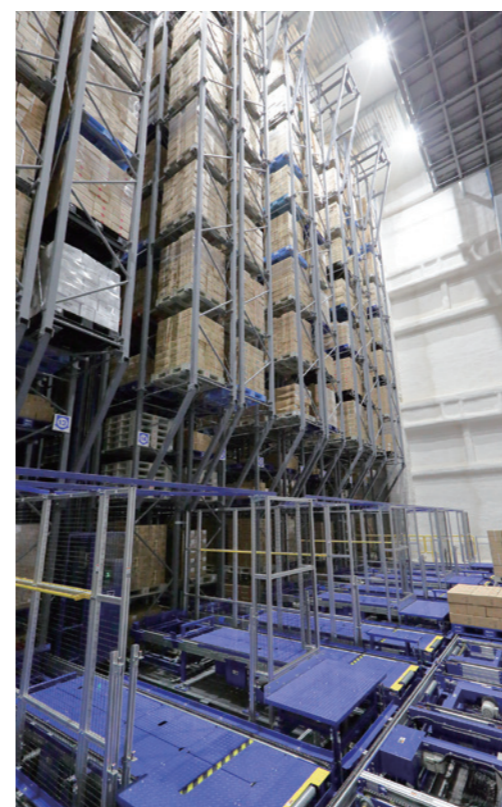
Automated freezer warehouse with storage for 7,000 racks
